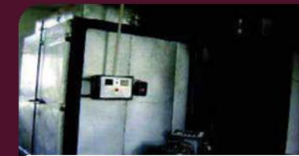
Powder Coating Unit
